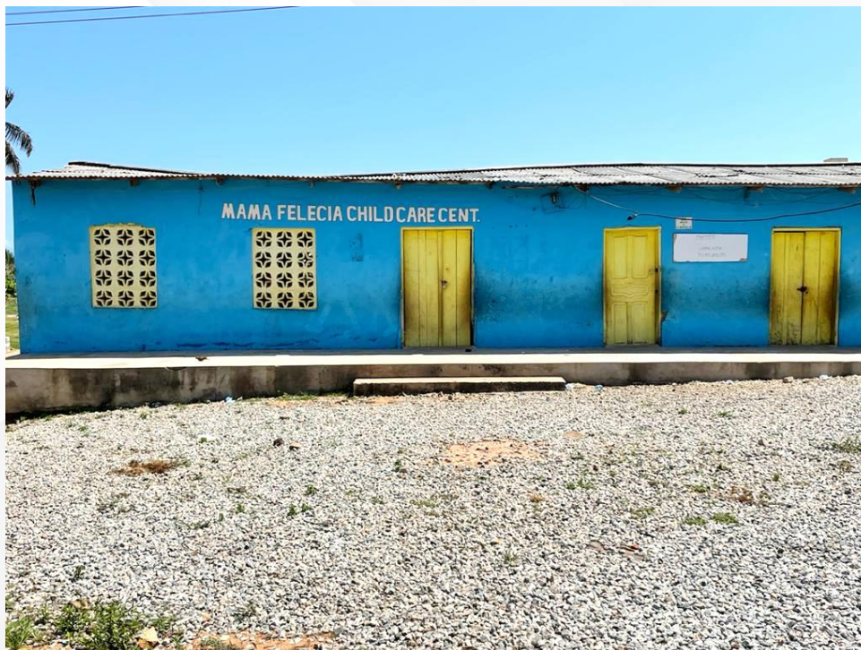
Mama Felicia Child Care Center - A Collapsed LCPS in Bortianor in the Ga South District.
